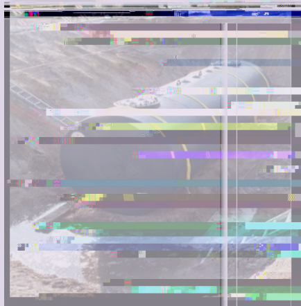
UST with hold down straps on a concrete pad Credit: EPA
